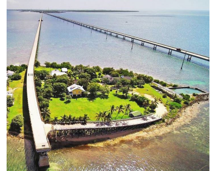
Coastal Florida bridges both large and small are vulnerable to chloride penetration and corrosion.
