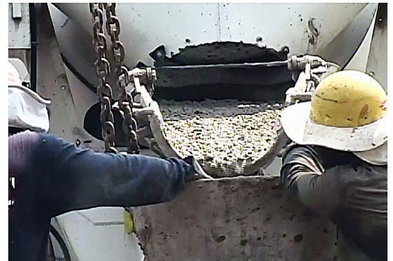
Concrete pours from truck to mold. Workers often work closely with concrete, possibly for hours at a time, increasing exposure to potentially harmful ammonia.
