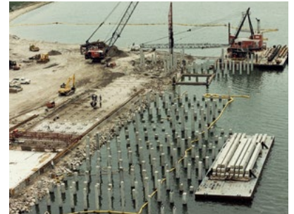
Piles loaded on a barge wait to be driven as a foundation for a Tampa-area pier.
