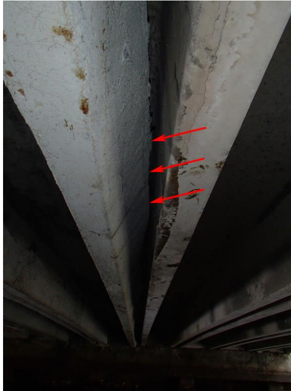
Figure 65—Debonded FRP wrap on a double tee girder
