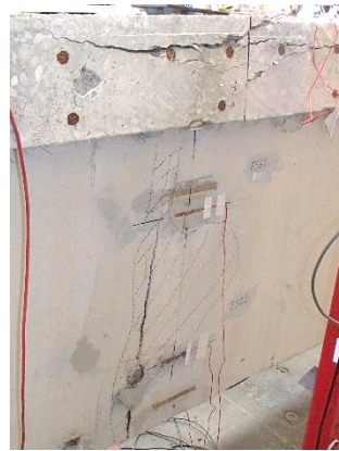
Figure 192—GFRP rupture and GFRP debonding indicated in hatch (Girder 3-2)
