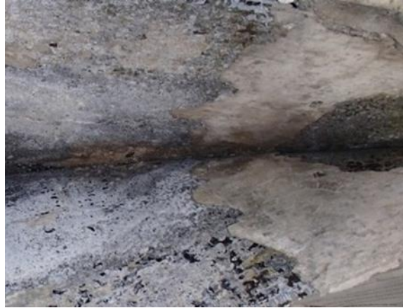
Figure 121—Evidence of skim coat at the bond
