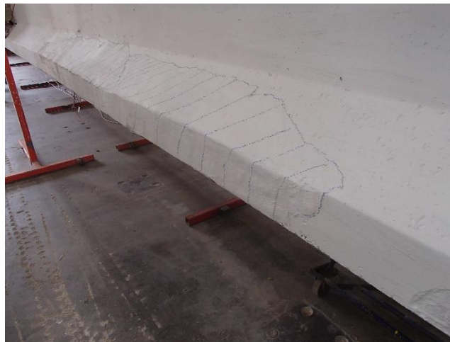
Figure 245—Region of concrete repair indicated in hatched area
