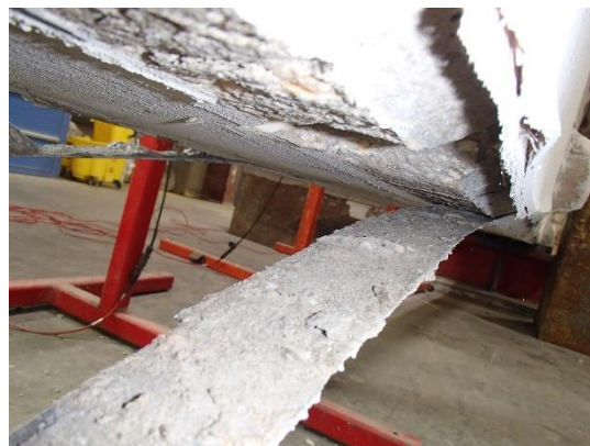
Figure 177—Debonded CFRP strips (Girder 4-1)
