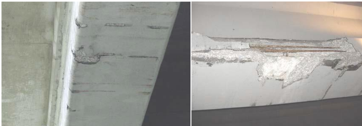
Figure 229—Condition of girder before and after vehicle impact in June of 2003
