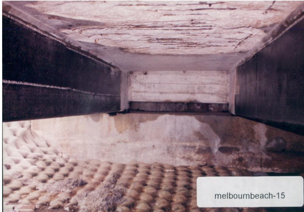
Figure 130—Example of wetting caused by wind and wave action
