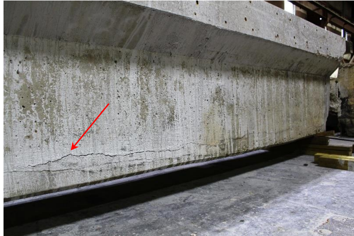
Figure 143—Horizontal crack on Girder 3-1 indicated by red arrow
