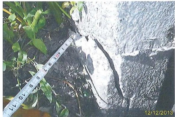
Photo #2 Element 204 - Pile 3-5 fracture in south face
