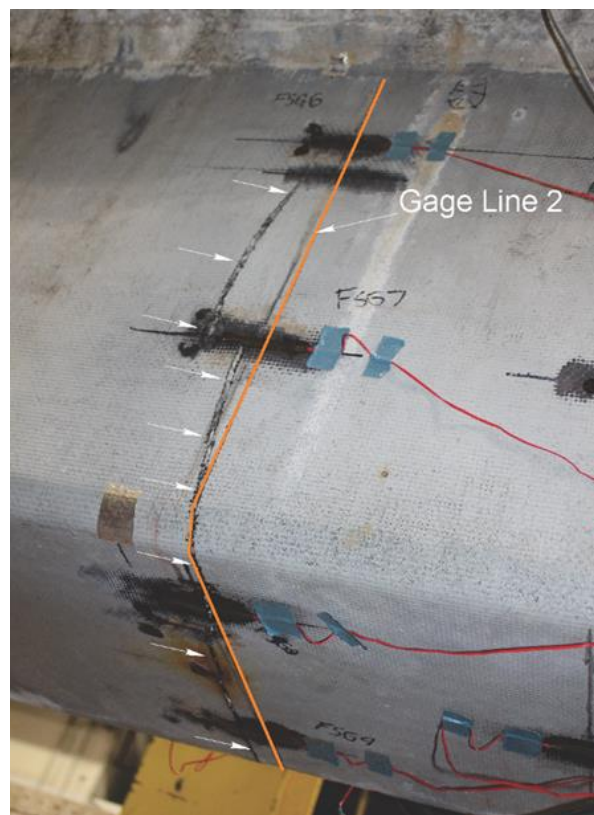
Figure 117—CFRP rupture relative to Gage Line 2 on Girder #1
