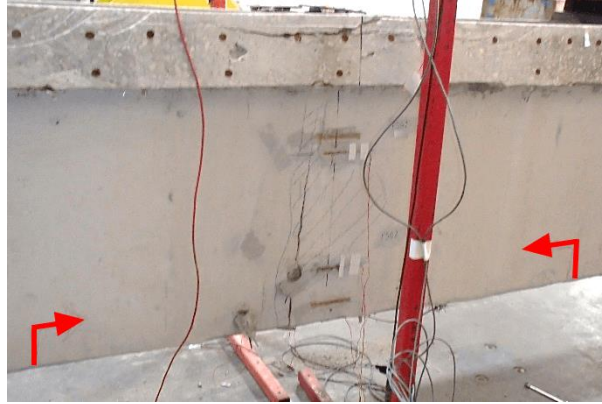
Figure 191—Red arrows indicate the span of debonded CFRP strip (Girder 3-2)
