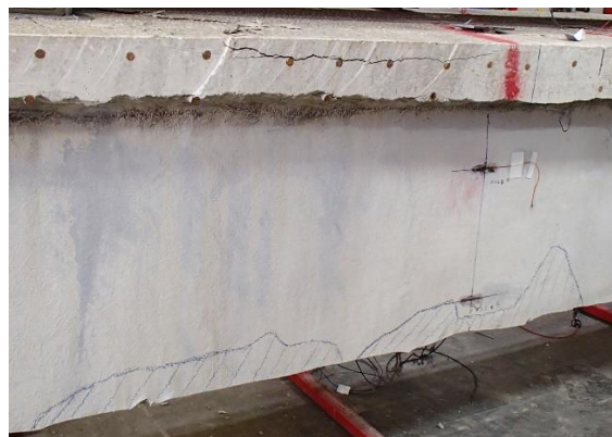
Figure 195—GFRP debonding by midspan on west elevation (Girder 4-2)
