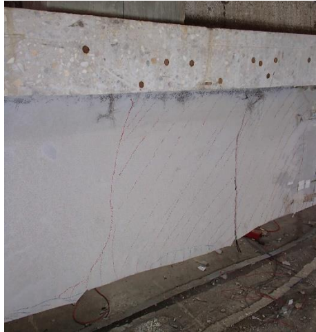
Figure 184—GFRP rupture (Girder 4-4)
