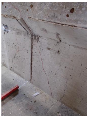
Figure 188—Formwork joint on the east elevation (Girder 5-1)
