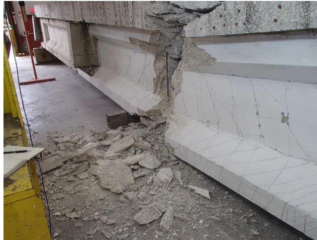
Figure 247—Girder 1 failed at the end of the repaired region
