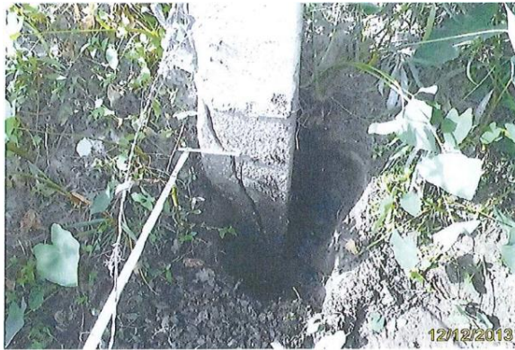
Photo #1 Element 204 - Pile 3-5 fracture in east face
