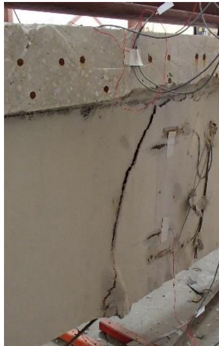
Figure 197—GFRP rupture on east elevation (Girder 4-3)
