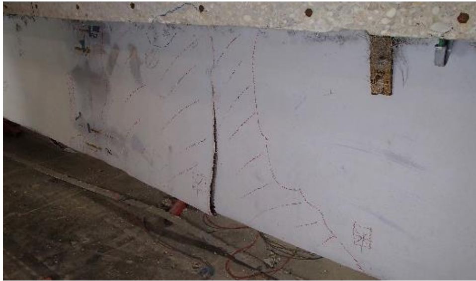
Figure 174—GFRP rupture (Girder 3-4)
