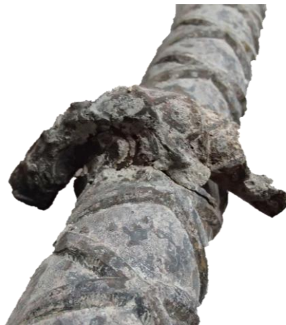
Figure 147—Stirrup remaining on steel reinforcement sample
