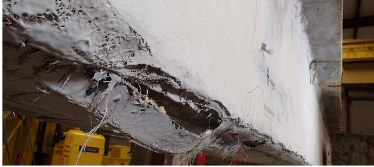
Figure 173—CFRP debonding (Girder 3-4)
