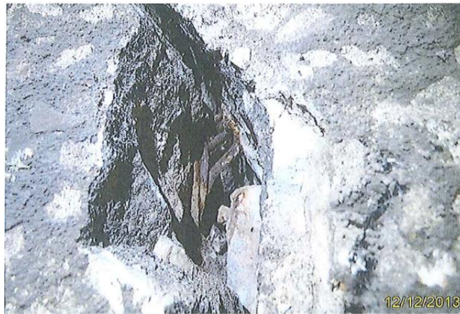
Photo #5 Element 204 - Pile 3-5 exposed and corroded prestress strand (visible through east face)
