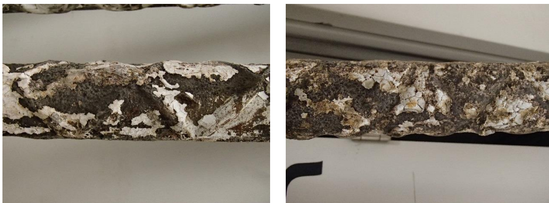
Figure 126—Close-up images of corroded reinforcement
