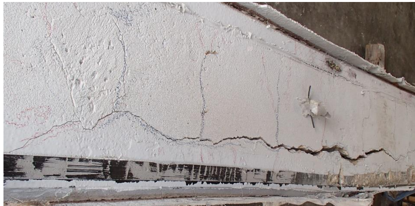
Figure 199—Longitudinal cracking on the tension face of Girder 4-3
