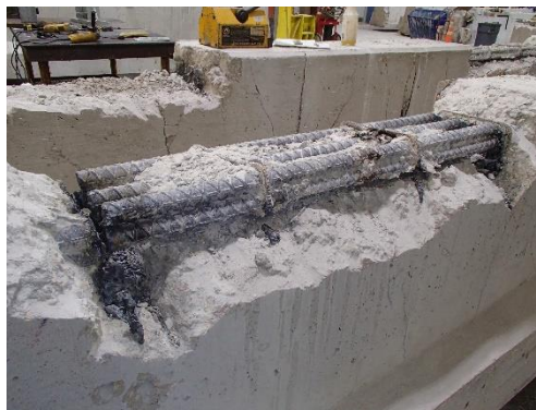
Figure 210—Steel reinforcement exposed
