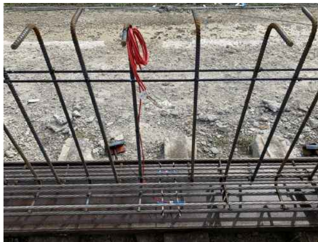
Figure 6-18 VWSGs attached to the bottom layer of HSSS strands in Girder E1
