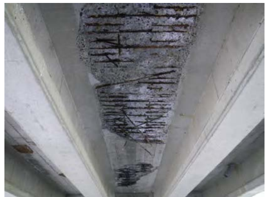
(b) Destruction of transverse reinforcement
