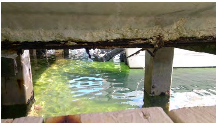
(a) Destruction of longitudinal reinforcement
