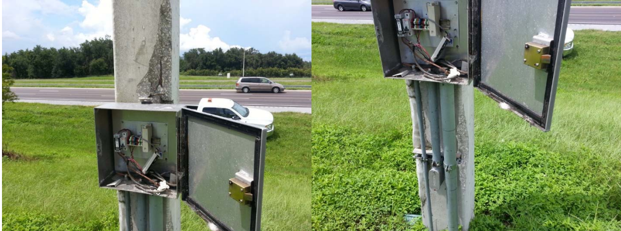
Figure 4.8. Direct Lightning Strike Damage to MVDS site at MM 15.8 on I-4
