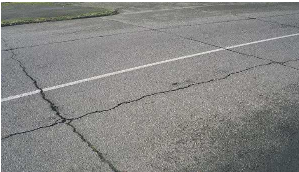
Figure 1.1. Reflective Cracking of Asphalt Concrete Pavement (from http://www.pavementinteractive.org/article/reflection-cracking/ )
