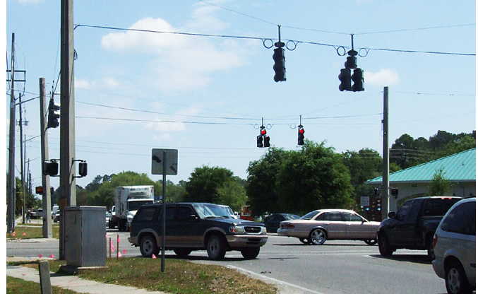
Above: The unobtrusive traffic control box at the left of this image integrates timing schedules, crossing request buttons, and in-road sensors to improve the efficiency and safety of intersections.
