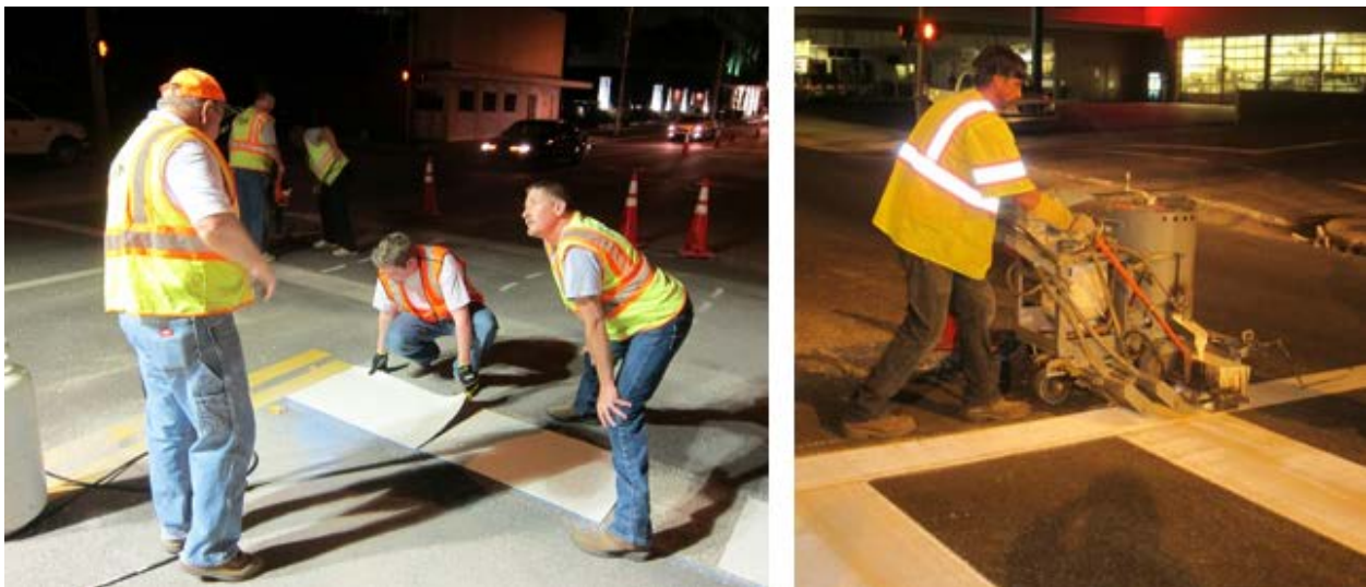
Figure 18. Installation of special emphasis crosswalk markings at Monroe and Carolina. Photos courtesy of Mary Anne Koos.
