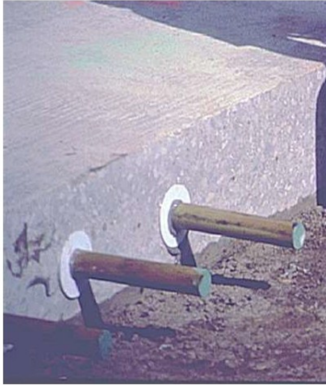
Figure 8.19: Insert new dowel bars fitted with a retention disk to prevent epoxy leak
