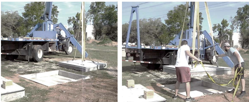
Figure 6.14: Use of a four-sling-lift method and a boom crane at FAMU-FSU test site
