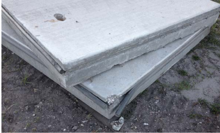
Figure 6.18: Damage to one of the precast panels during removal
