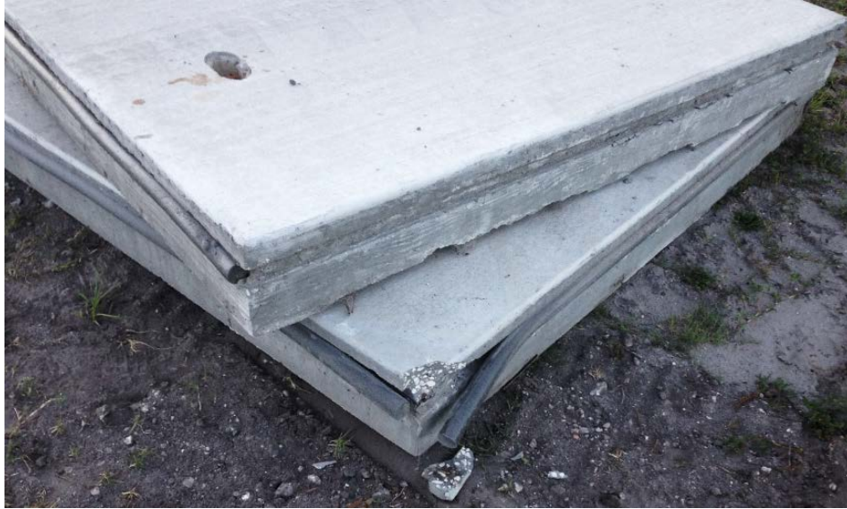
Figure 8.26: Damage to panel corner and stripping of backer rod gasket
