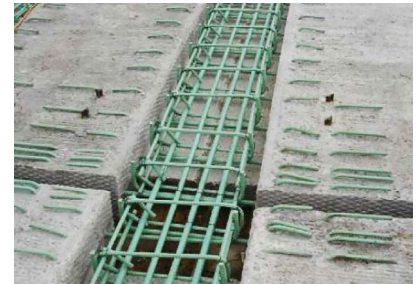
Steel protruding from adjacent FSB slabs and a steel cage form a joint between slabs when concrete is poured.
