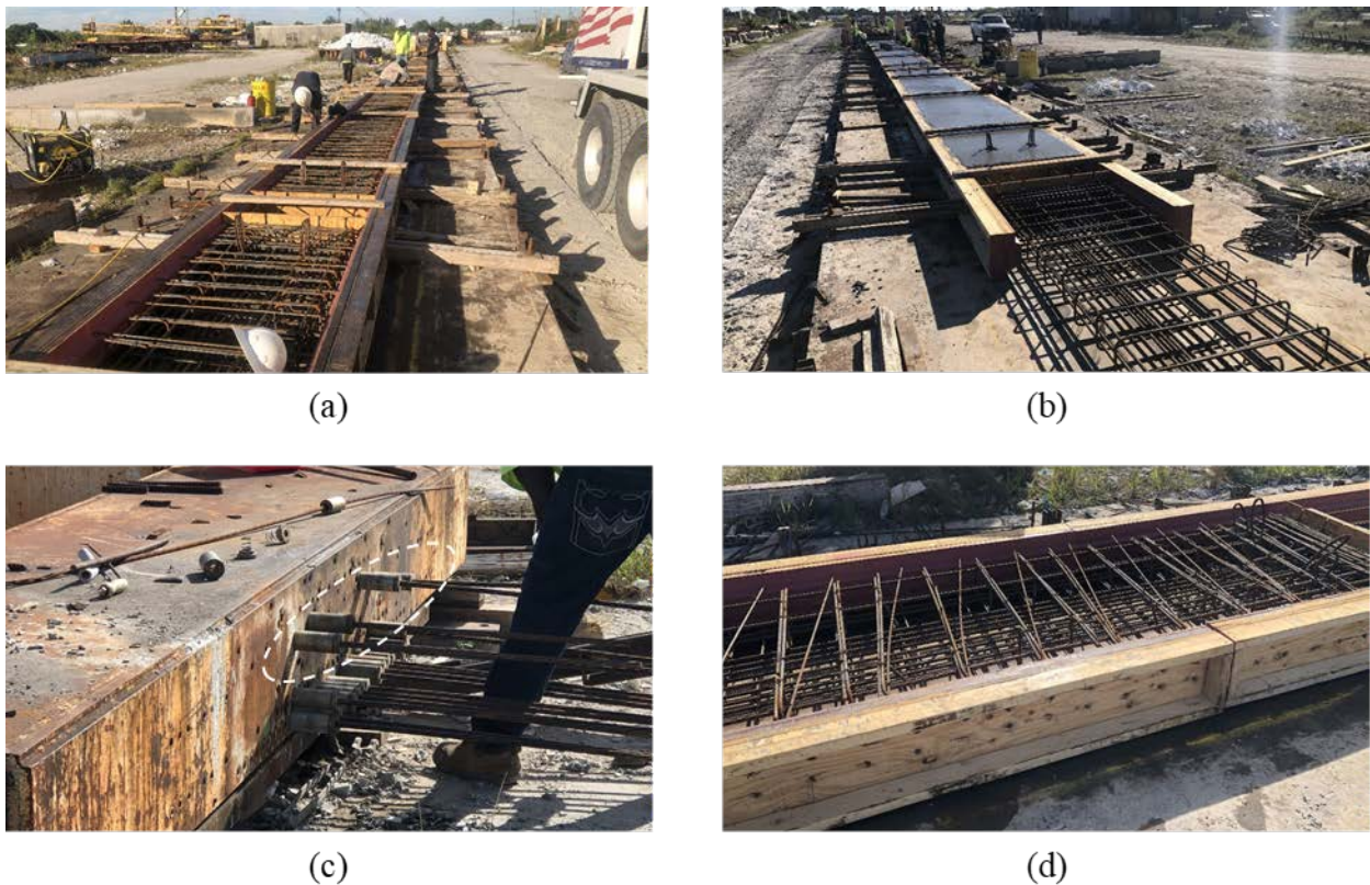
Figure 8.5: Construction of second set of beams: (a) FIU-8, FIU-7, and FIU-6 mild reinforcement and formwork construction, (b) concrete pour of first group of beams, (c) top strand layer de-tension, and (d) observed misalignment of mild reinforcement in second group of beams
