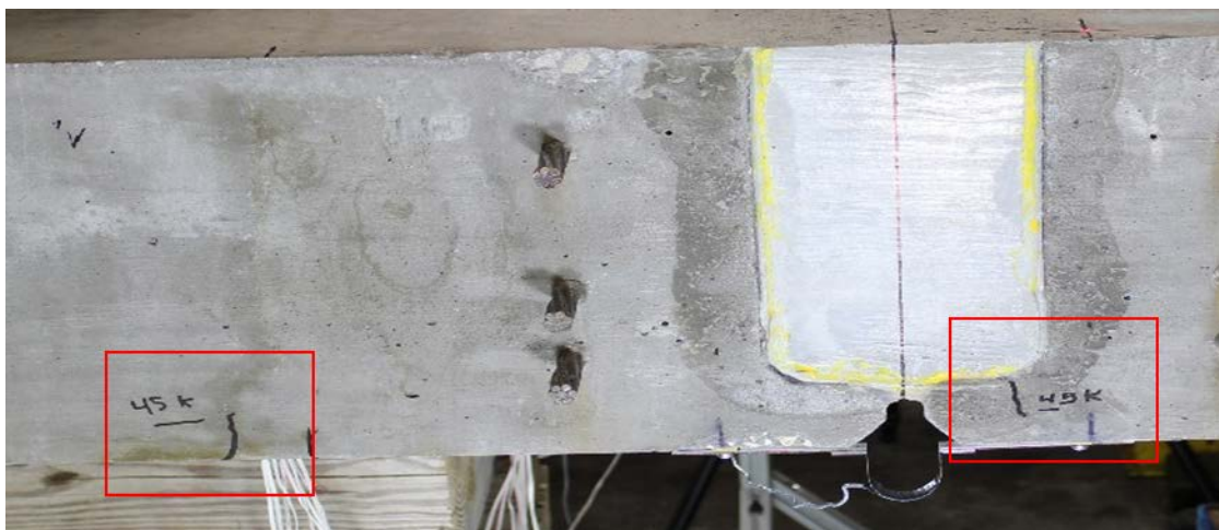
Figure 5.42: Actual cracks from visual inspection (12F2-1 shown)
