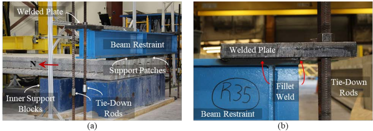
Figure 7.26: End moment restraint detail: (a) south-end view and (b) welded plate detail
