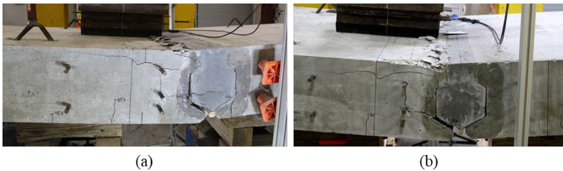
Figure 6.23: Failure crack for ultimate strength testing of 12A2 (a) without any fatigue load applied, 12A2-1 and (b) after fatigue loading, 12A2-2
