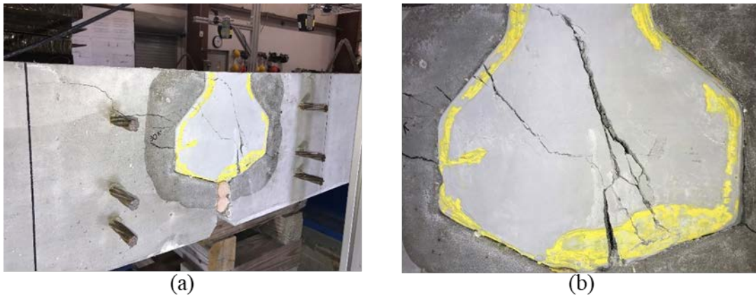
Figure D.46: 12A1-1: (a) failure cracks and (b) diagonal crack in UHPC matrix
