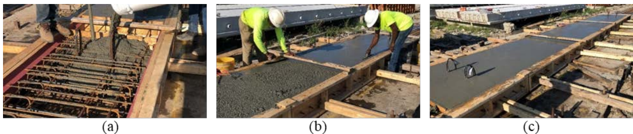
Figure 7.7: Casting of concrete for full-scale beams: (a) casting of concrete, (b) float finish on top of beams, and (c) finished beam after casting
