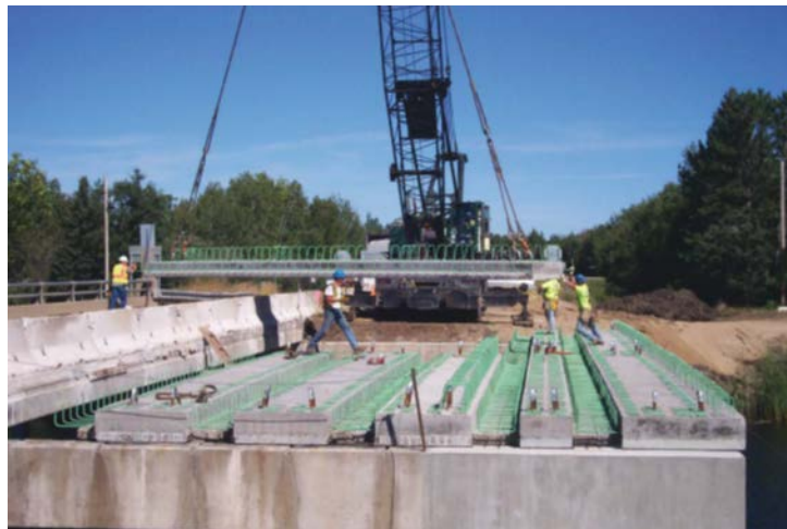
Figure 2.16: Erection of Bridge 04002 located on MN Highway 72 over the Tamarac River near the rural, northern Minnesota town of Waskish [11]
