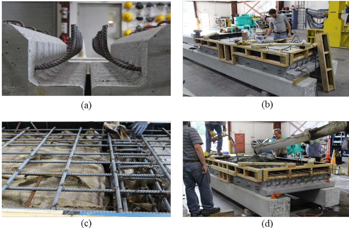
Figure 5.11: Construction of deck and joint in FSB: (a) adjacent FSBs with 3/4" spacing, (b) CIP deck form construction, (c) slab and joint reinforcement, and (d) CIP deck pour
