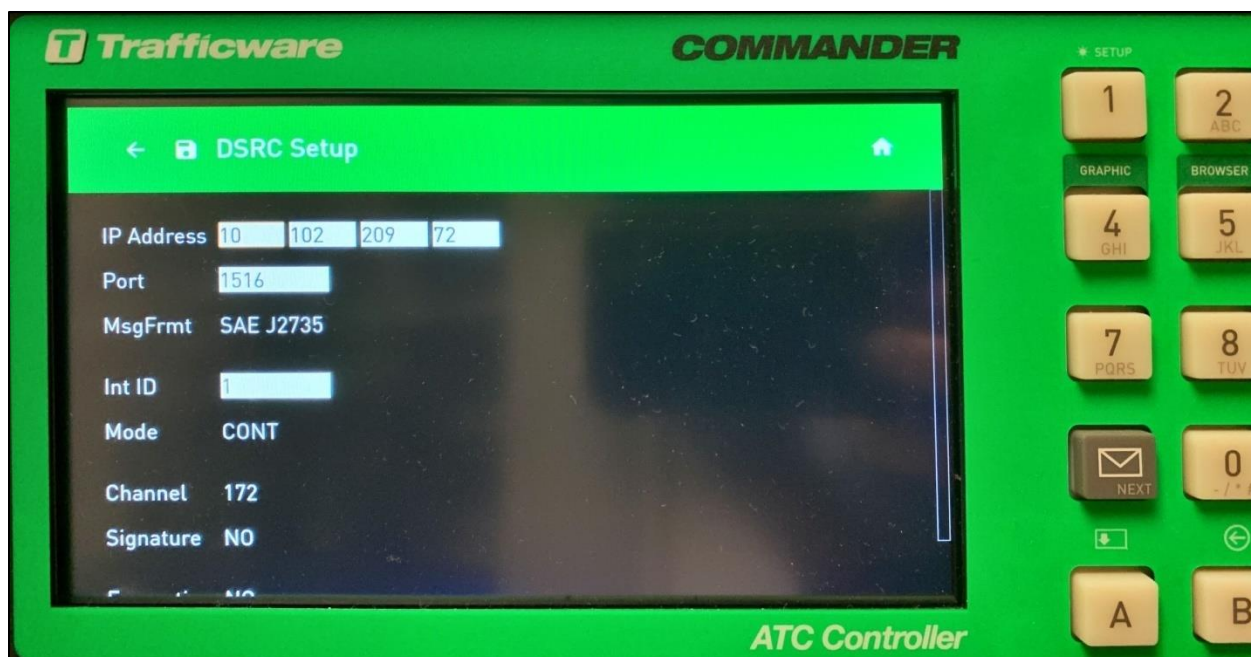
Figure 8-5 J2735 SPaT Configuration of TrafficWare Commander ATC Controller
