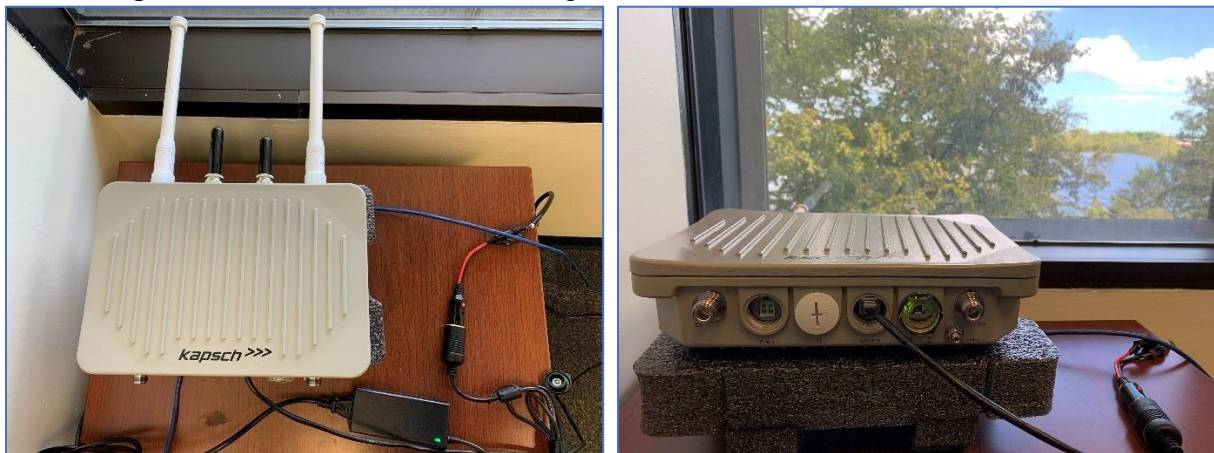
Figure 8-2 Kapsch RIS-9260 Roadside Unit
