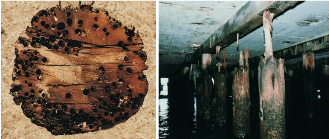
Figure 1: Tunneling in a timber pile caused by Teredo and Bankia (left), untreated timber piles attacked by Limnoria (right) [16]
