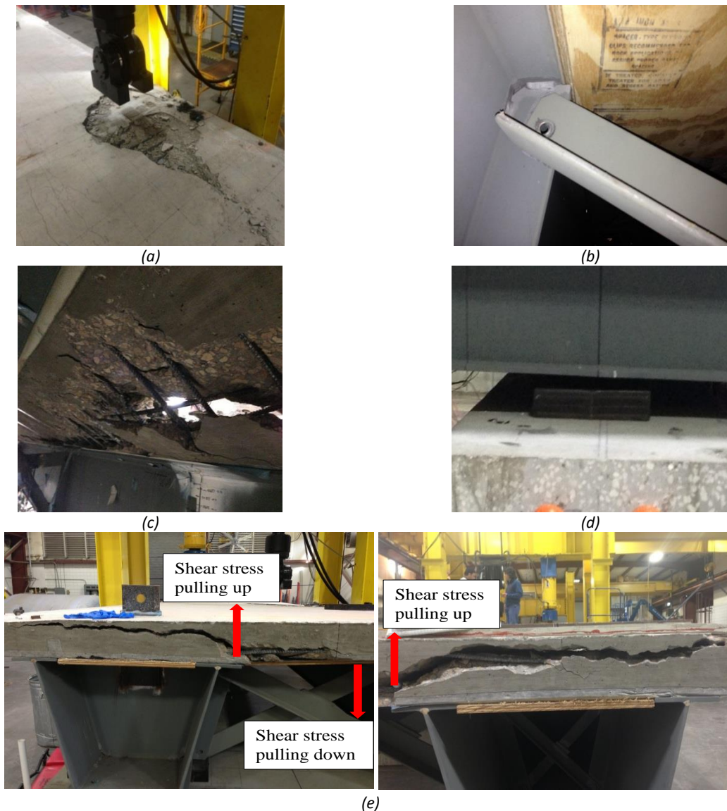
Figure 5-24. Damages in the Test E-1 of FIU bridge.
