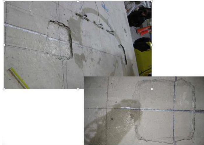
Figure 5-25. Punching shear failure in the Test E-2 of FIU bridge.
