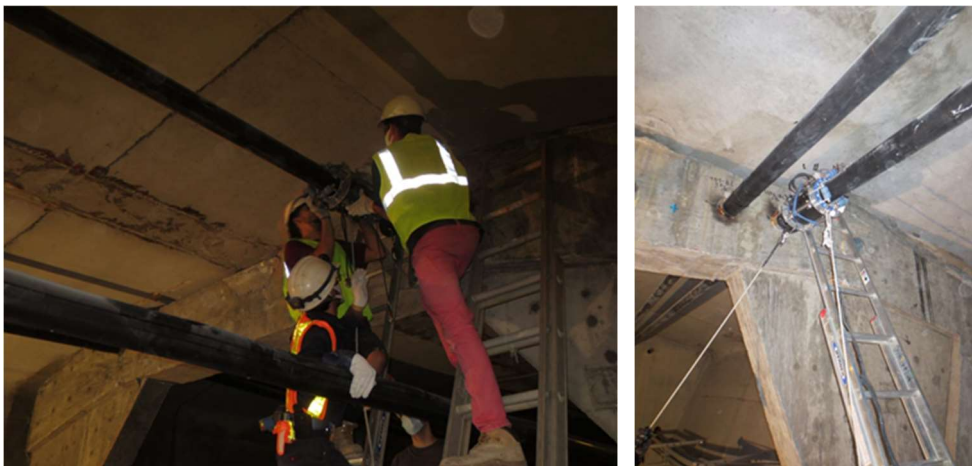
Figure 4-2: MMFM testing on external PT tendons.
