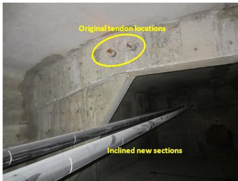
Figure 19. Two replaced tendons that bypassed an upper deviator.
