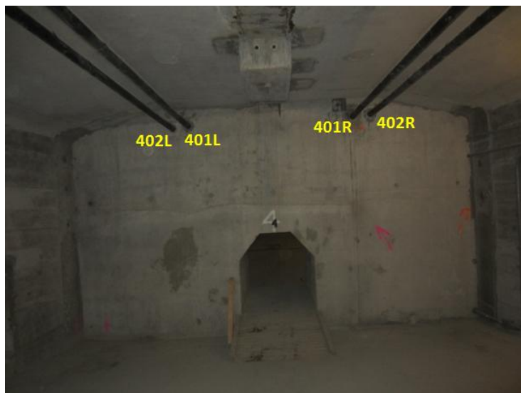
Figure 16. Typical tendon arrangement in the center cell (west face of pier 4 diaphragm).
