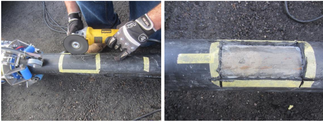
Figure 12. Making a 6 x 3 inches duct opening (left) and as-exposed grout condition (right).
