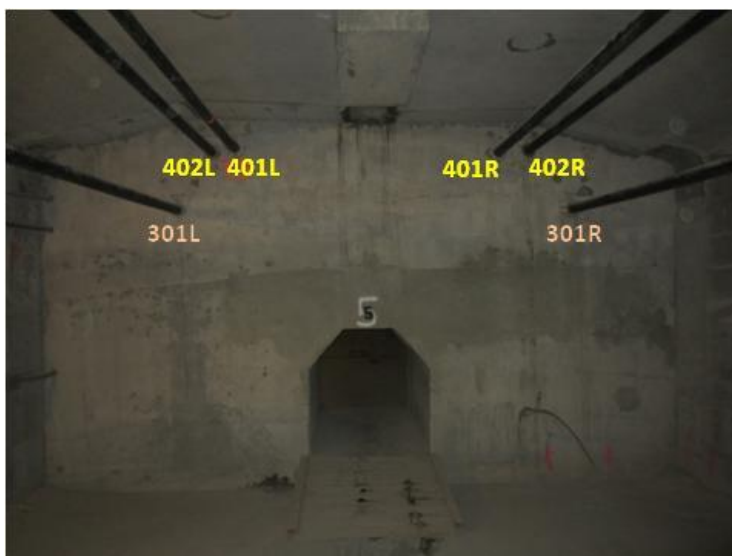
Figure 17. Tendon arrangement having two extra tendons in the center cell (east face of pier 5 diaphragm).
