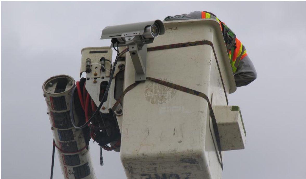
Figure 4-6. ITERIS Camera Installed on Bucket
