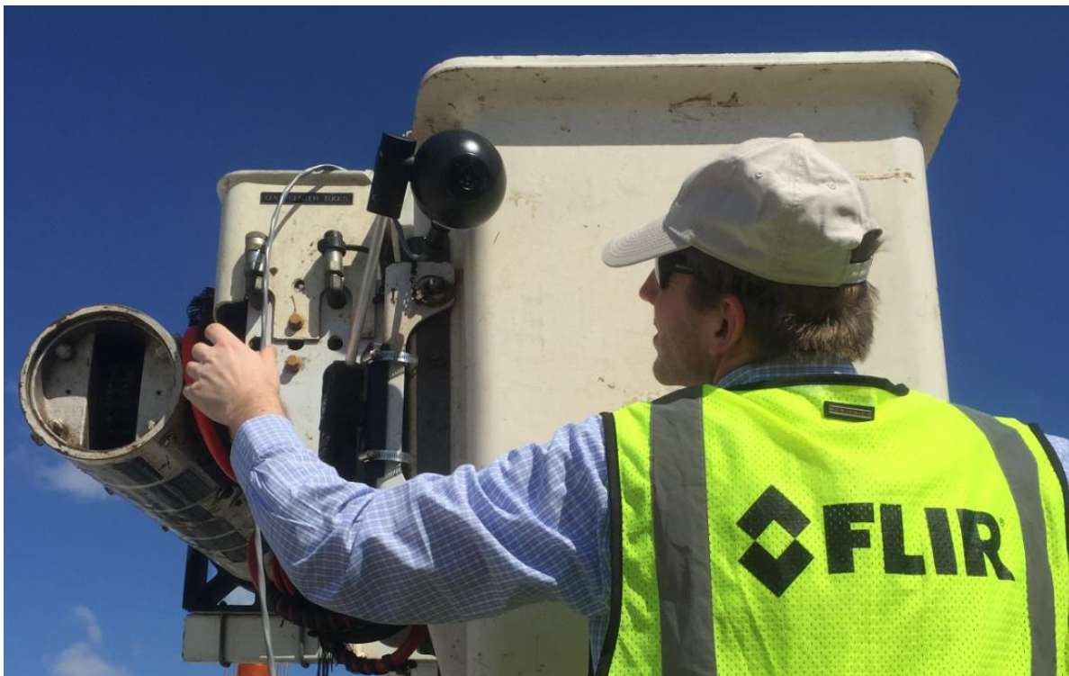
Figure 4-10. FLIR Camera Installed on Bucket
