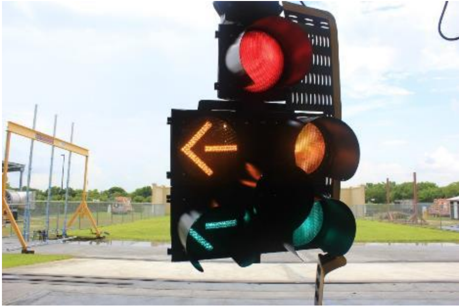
Figure 40: The 5-section signal with damaged back plates and visors
