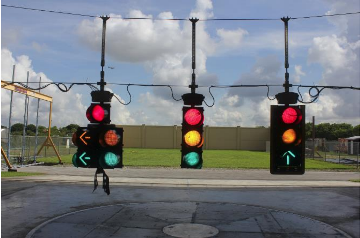
Figure 72: Traffic signals after 30 to 130 mph wind speeds test
