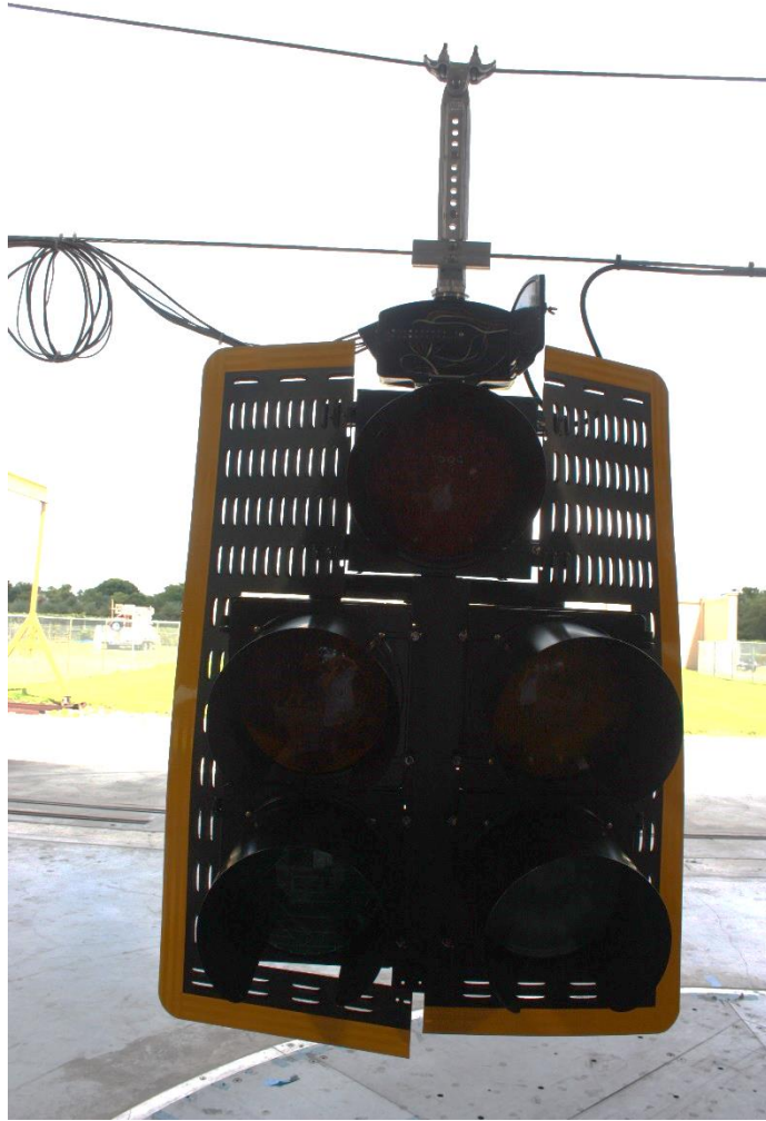
Figure 102: 5-Section signal with damaged back plates
