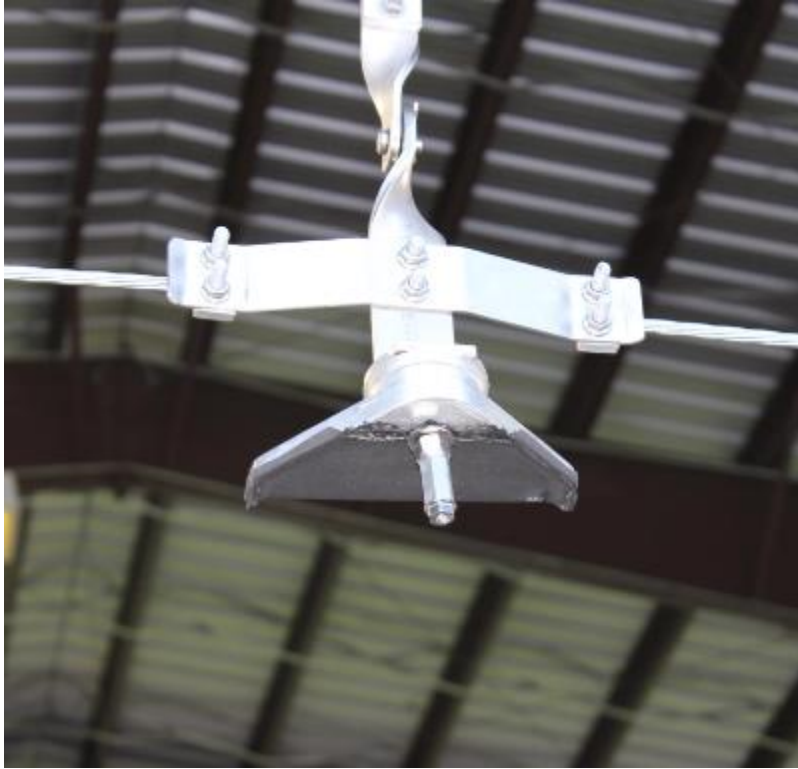
Figure 58: East 3-section signal hanger attachment
