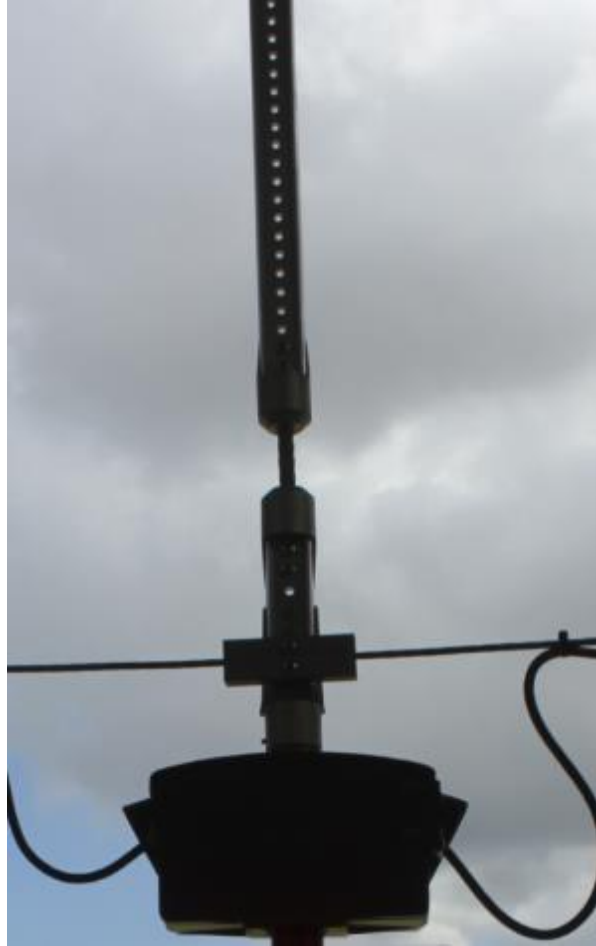
Figure 71: Pelco adjustable hanger assembly with cable dampener after full range test
