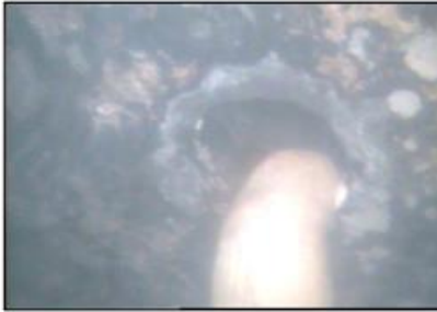
Figure 3.2. Underwater Image of a Hole on a Steel Pile due to Corrosion. Photo courtesy of FDOT.
