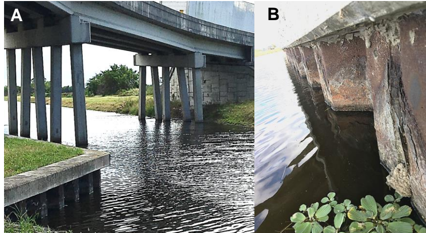
Figure 3.25. Images of Turnpike/Boynton Beach Site (west side) (Site 5). A. View of the site. B. View of corroded steel piles.
