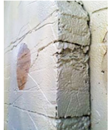
Serious cracking can be observed in this epoxy pourback, which encases a post tensioning anchorage (marked by the dark spot).
