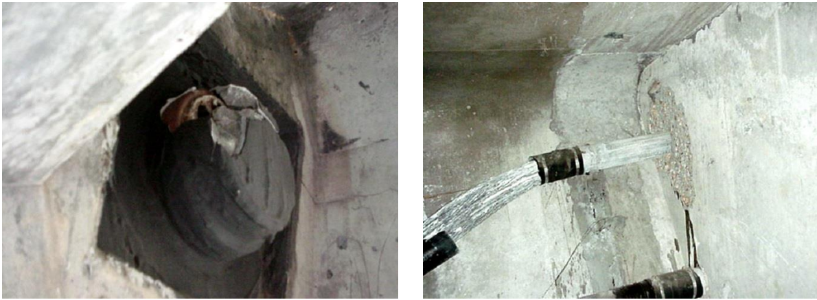
Figure 1-1: Tendon failure on the Mid-Bay Bridge
