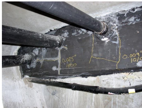
Figure 1-2: Pourback cracking on the Sunshine Skyway Bridge
