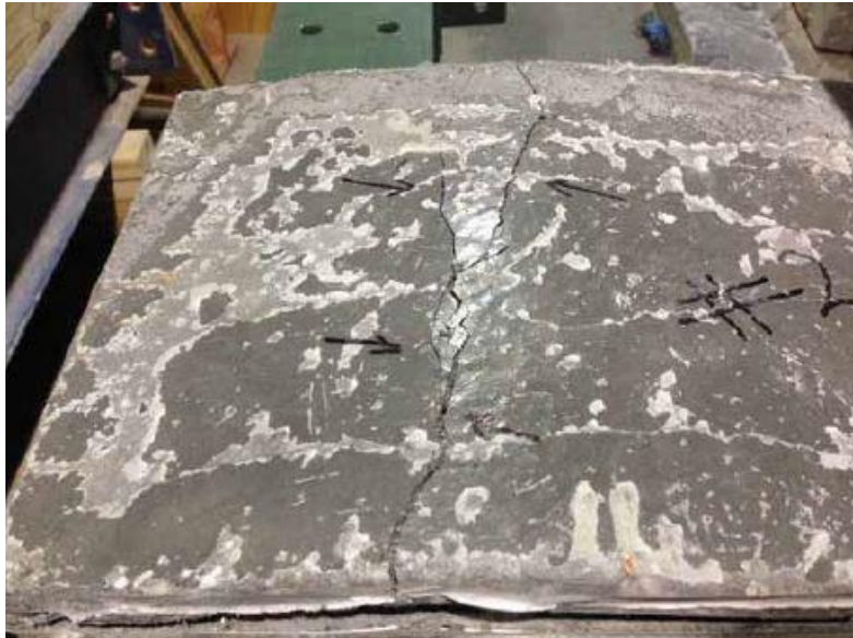
Figure 4.12 Failure Mode near the End of the Grouted Region
