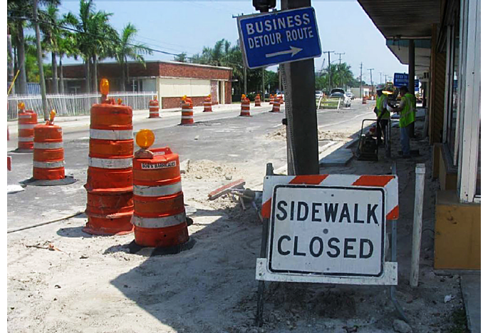
Road construction can disrupt bus routes and safe access to bus stops.
