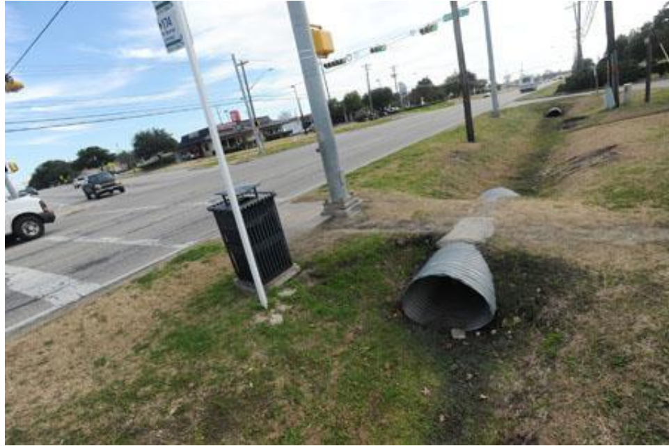
Figure 5-19: Bus Stop near a Drain Pipe
