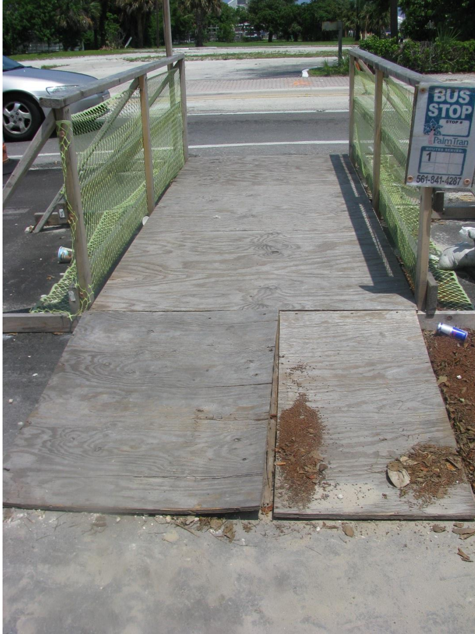
Figure 7-4: Poor Conditions of Temporary Bus Stop
