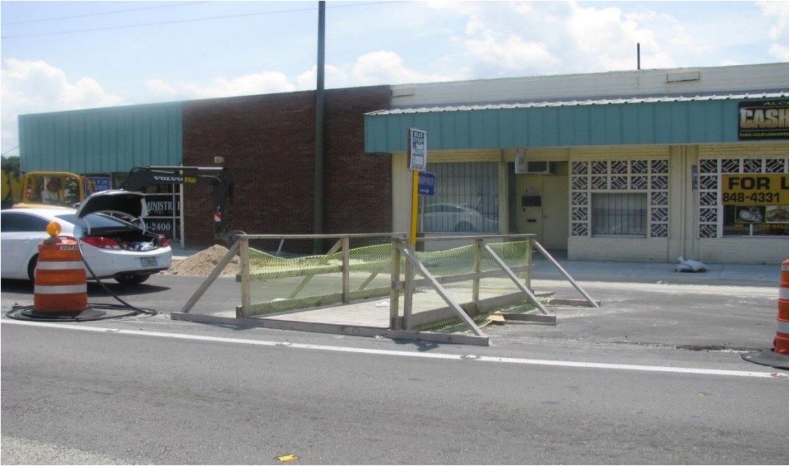
Figure 5-16: Non-Compliant Pedestrian Platform
