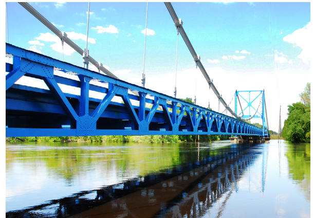
This steel bridge depends on its bright blue coating to protect it from corroding in its moist environment.
