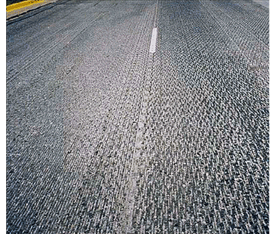
Asphalt removed by milling can be recycled and reused to pave again.
