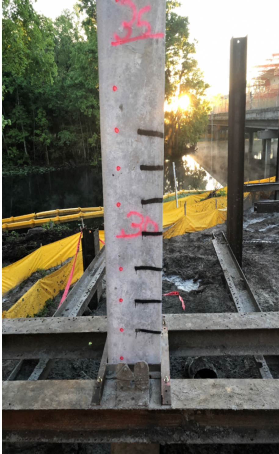
Figure 3-25 Photo of Wekiva Bridge 110118 Pier 8, Test Pile 1 with black paint for CMS Evaluation
