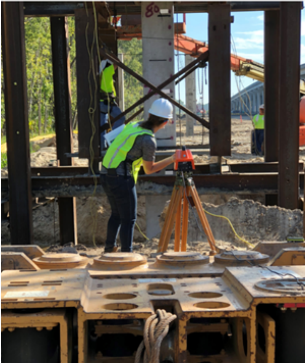
Figure 6-8 Images of Pile and PDM Setup for Dunns Creek (Photo by Dr. Bostater)
