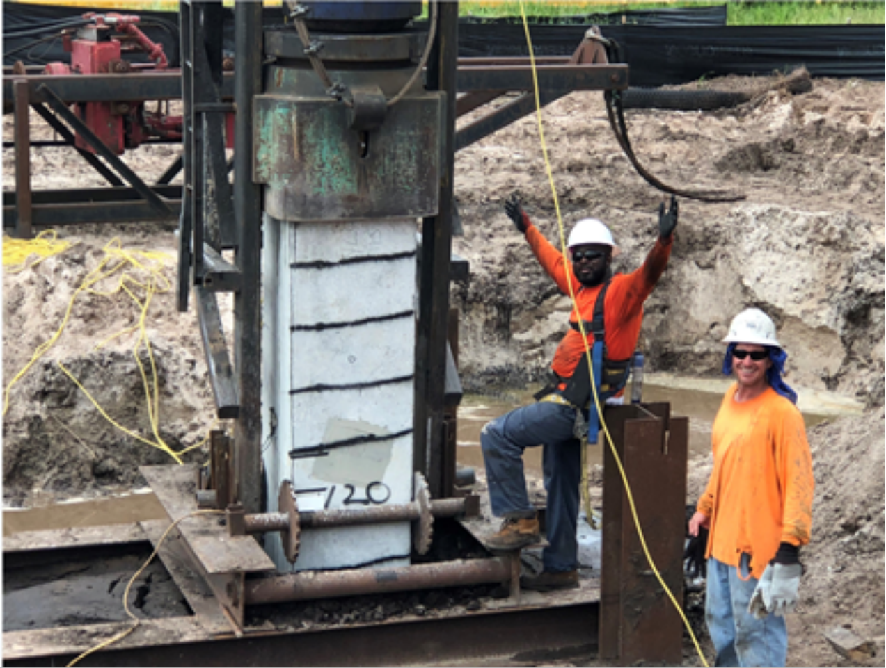
Figure 6-6 Images of End Bent 1, Pile 12 and PDM Setup for Reedy Creek (Photo by Dr. Cosentino)
