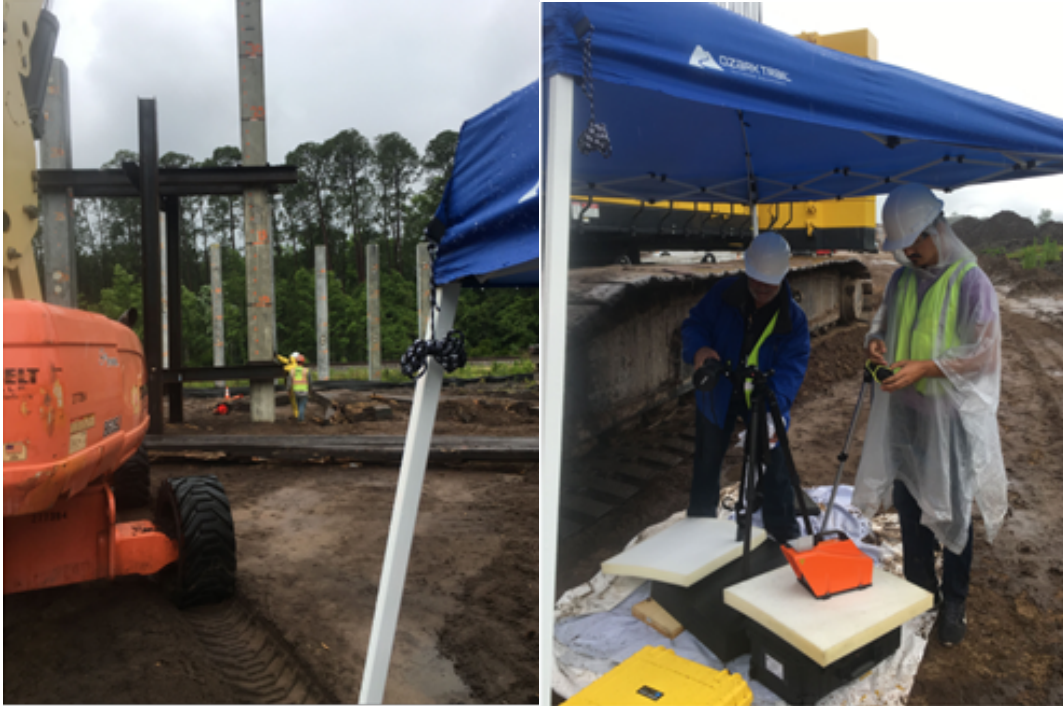
Figure 6-5 Images of Pile and PDM setup for Baldwin Bypass (Photos by Cosentino)
