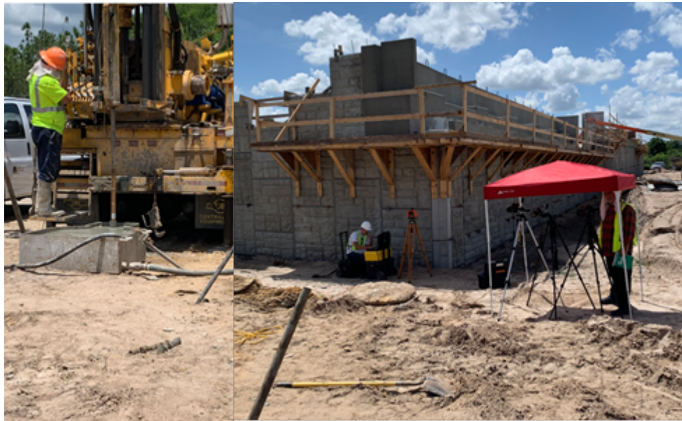
Figure 6-13 Images of SPT and PDM Setup for Wekiva Parkway WLC 3 Day 2 (Photos by Dr. Cosentino)
