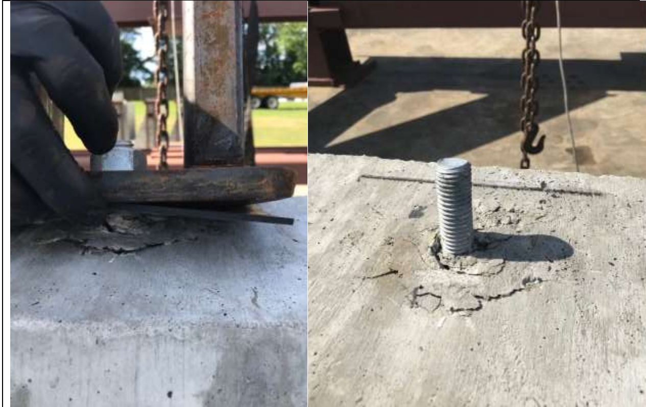
Figure 20: Adhesive Bond Failure in Gravity Wall with 12-inch Adhesive Anchor Embedment
