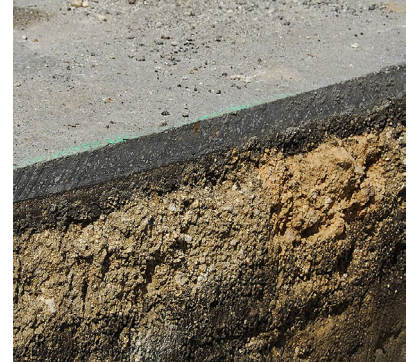
This pavement cross-section shows the asphalt surface supported by a layer of compressed aggregate and soil.
