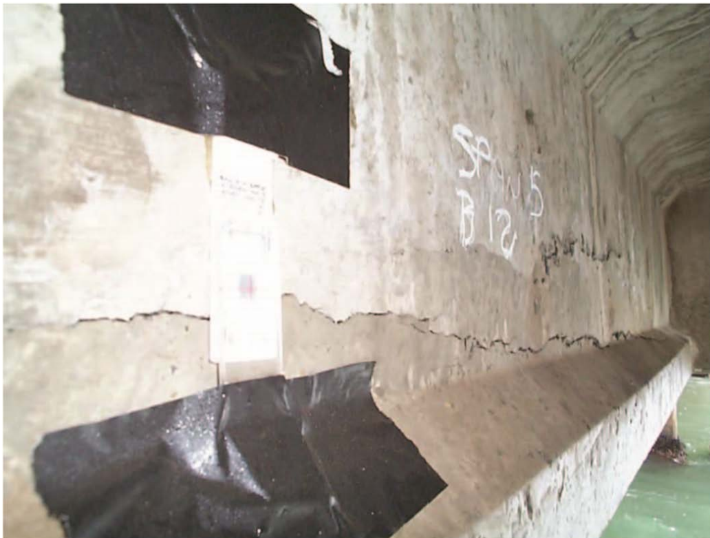
Figure 7. Typical longitudinal web crack along a beam [12]
