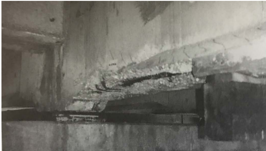
Figure 5. Corrosion damage on post-tensioned beam on Gandy Bridge [57]
