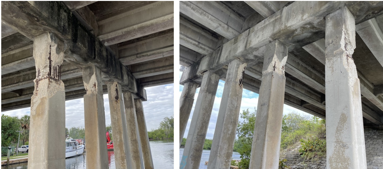
Figure 62. Bent 4, left image shows north face (piles P4-5 to P4-1), right image south face (P4-5 to P4-1)
