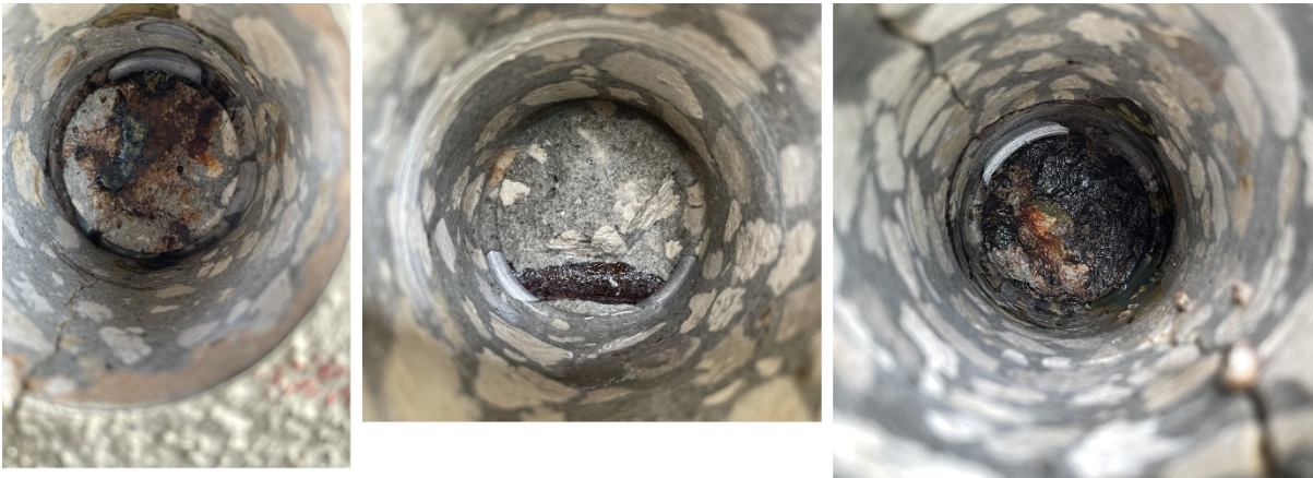
Figure 60. Pictures after removing cores in bent 8, left two images from east column, right west column.
