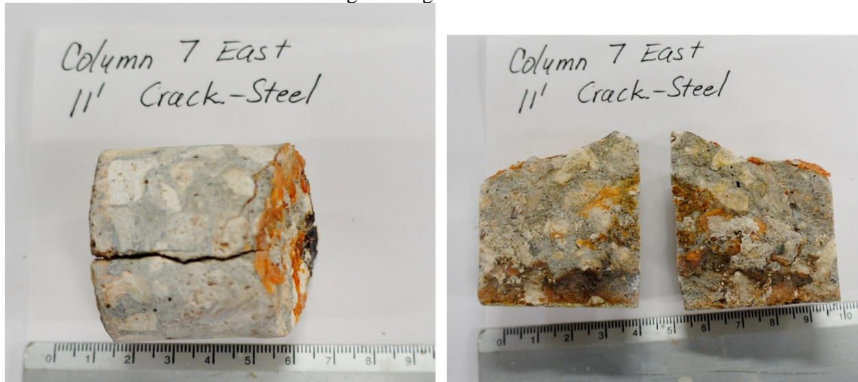
Figure 67. Core obtained column 7 at 11 ft above MHWL
