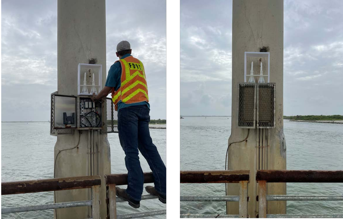
Figure 18. Wet candle setup installed on top of electric box, fishing area (elevation approx. 21 ft MHWL). (Core – fresh patch – was obtained at 22 ft MHWL)
