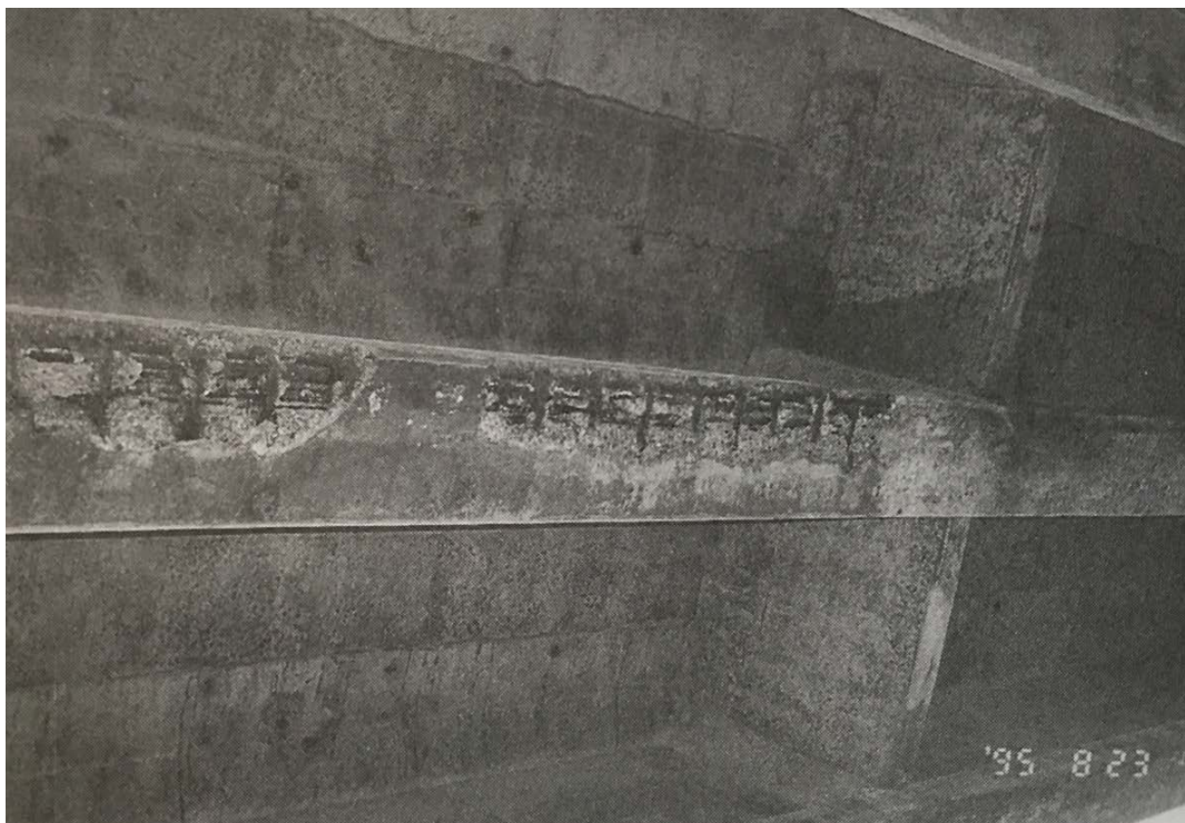
Figure 4. Corrosion damage on main girder on the bridge along the seashore of the Sea of Japan [55]
