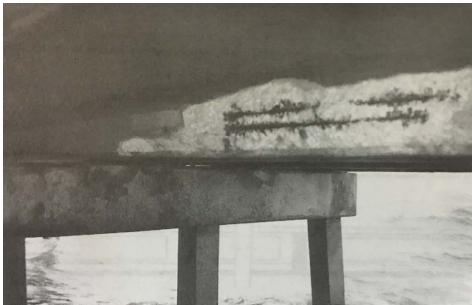
Figure 6. Spalled areas over pretension tendons on abutment span Old SSK bridge [57].
