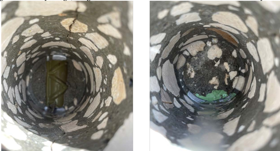
Figure 65. Bridge #100585, pictures taken after removing the cores, showing that reinforcement was reached
