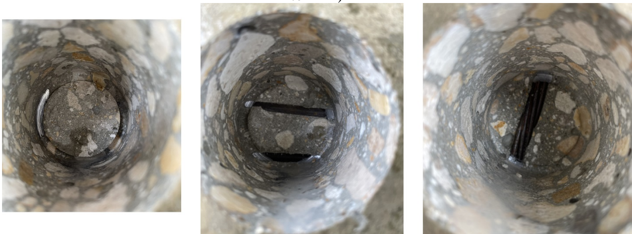
Figure 63. Pictures taken after removing the cores at the bridge in Dania Beach (bridge #860160).
