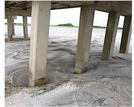
Flooding from a hurricane created heavy flows that created scours around the bridge supports.
