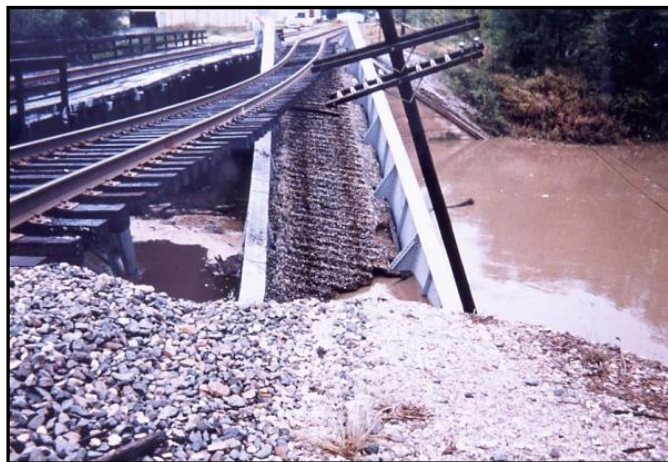
FIGURE 1-1. Example of a bridge washout due to stream instability and or scour (1)
