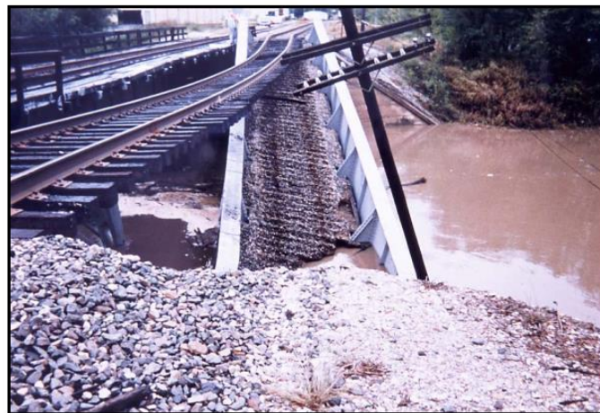
FIGURE 1-1. Example of a bridge washout due to stream instability and or scour (1)
