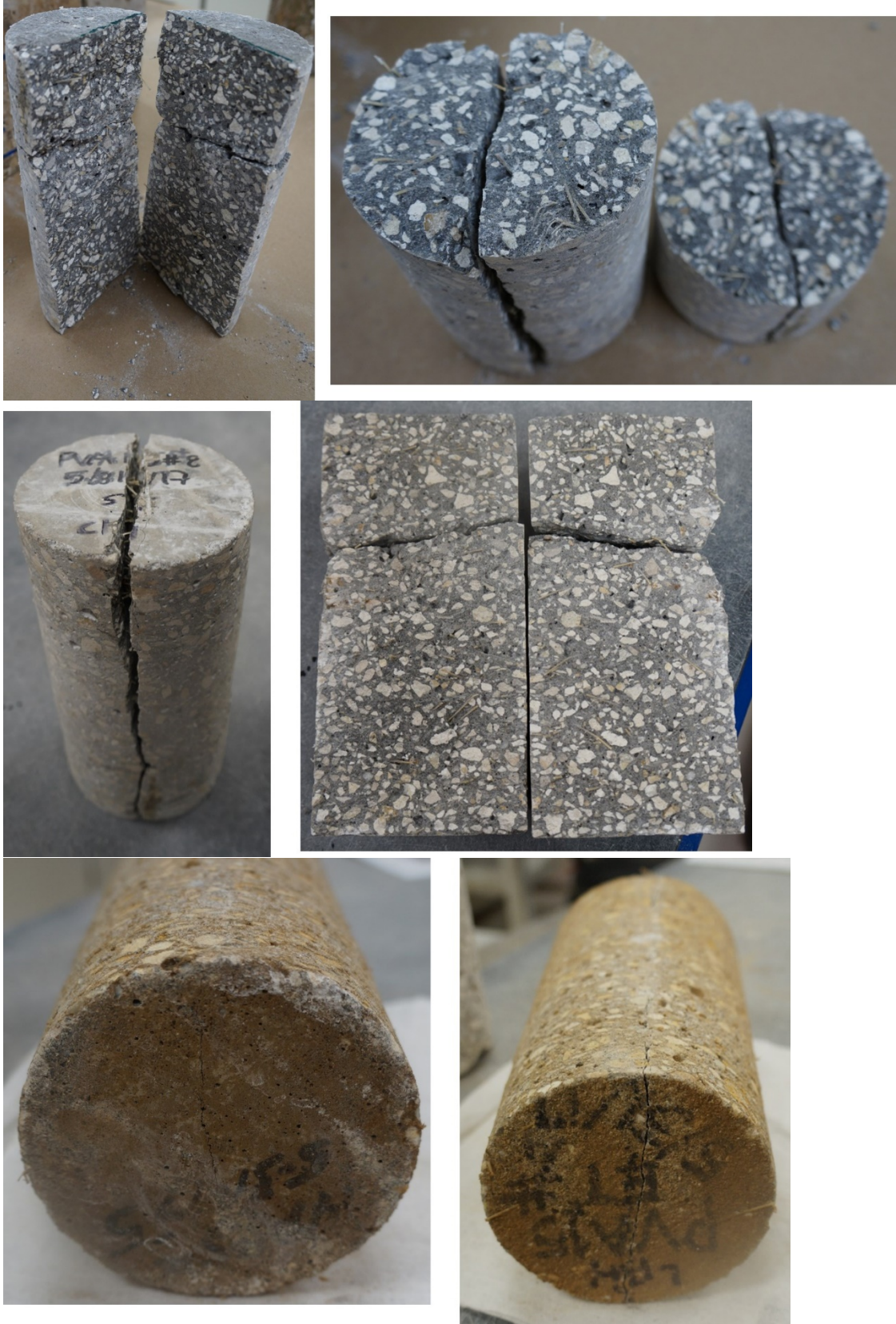
Figure 145. Visual inspection after split-tensile tests on cores of mix 6
