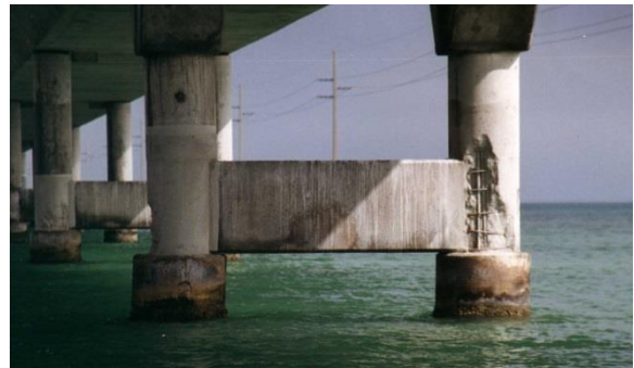
Figure 1: An example of corrosion damage caused by the diffusion of saltwater chlorides into concrete.
