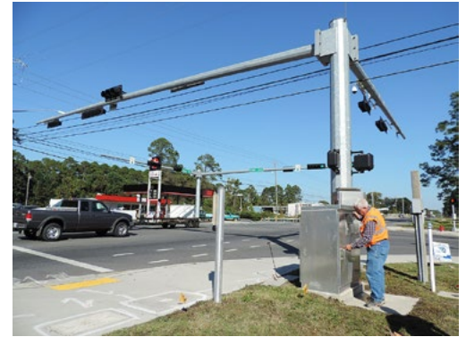
A worker accesses a traffic signal control cabinet.
