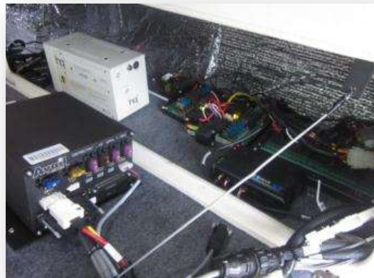
Figure 4-3: Vehicle Security Camera System on Collier Area Transit Fleet Vehicle
