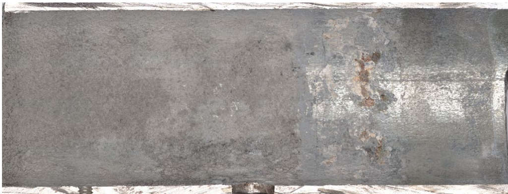
Figure 5-7. Inside view of the galvanized duct from Tendon 7 with semisoft grout (w/c = 0.38).
