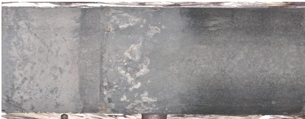
Figure 5-5. Inside view of the galvanized duct from Tendon 5 with very soft grout ( w/c = 0.5 ).
