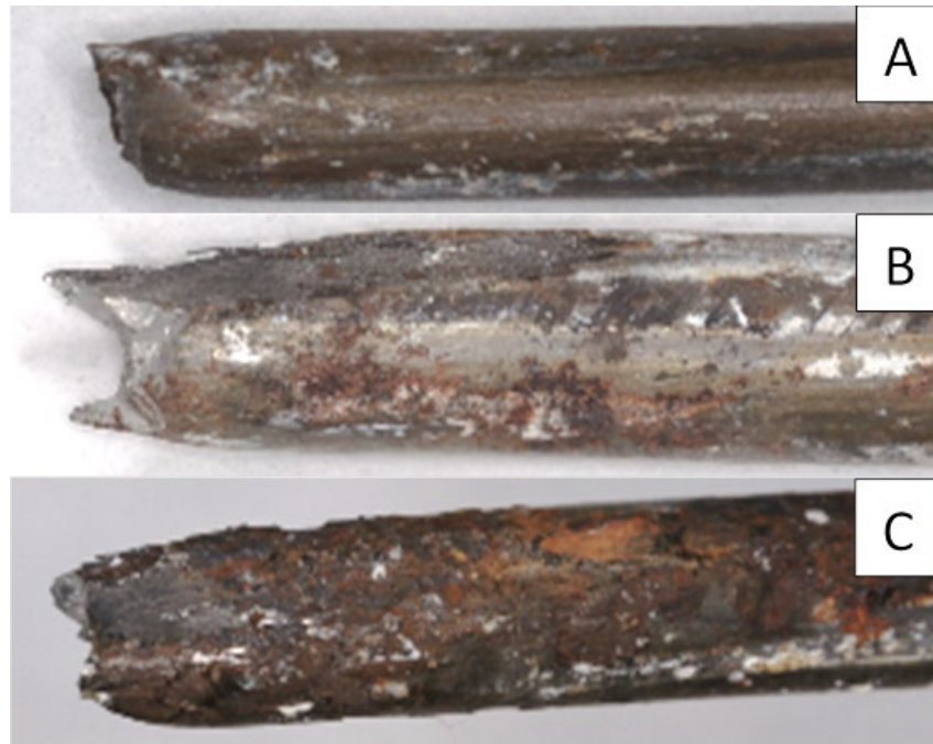
Figure 3-7. Example of (A) strands that have no corrosion, (B) mild corrosion, and (C) moderate corrosion.
