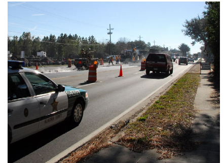
Work zones on arterials with a lane closure are one situation where workers and drivers are at extra risk.
