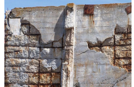
Preventing corrosion damage to concrete structures can eliminate or delay expensive repairs.
