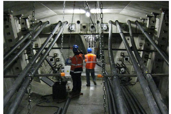
Workers inspect the post-tensioning cables that run through the inside of a box girder bridge.
