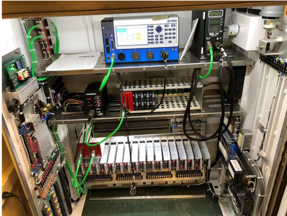
Figure 6.3 CUTR traffic cabinet donated by the City of Tampa
