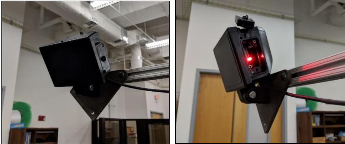
a) Installed on a pole
