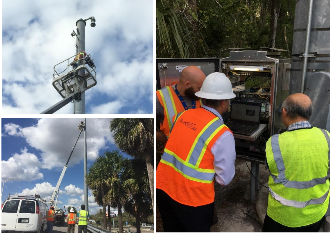
Figure 3-2 Field Installation of Fixed Cameras
