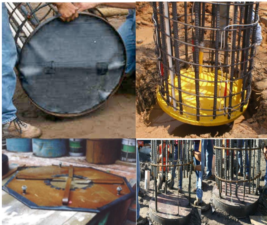
Figure 2.2 Flat jacks used in West Palm, FL (top left), Houston, TX (top right), Taipei, Taiwan (bottom left), and Tampa, FL (bottom right).
