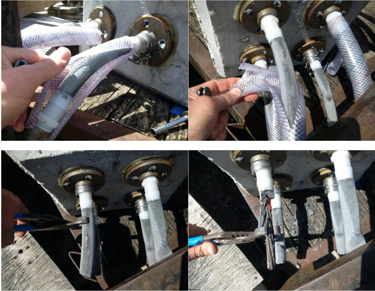
Figure 4-58: Removal of hoses (top); breaking grout off the strands (bottom) before installing new hoses and valves on both ends of the entire 8 specimen assembly.
