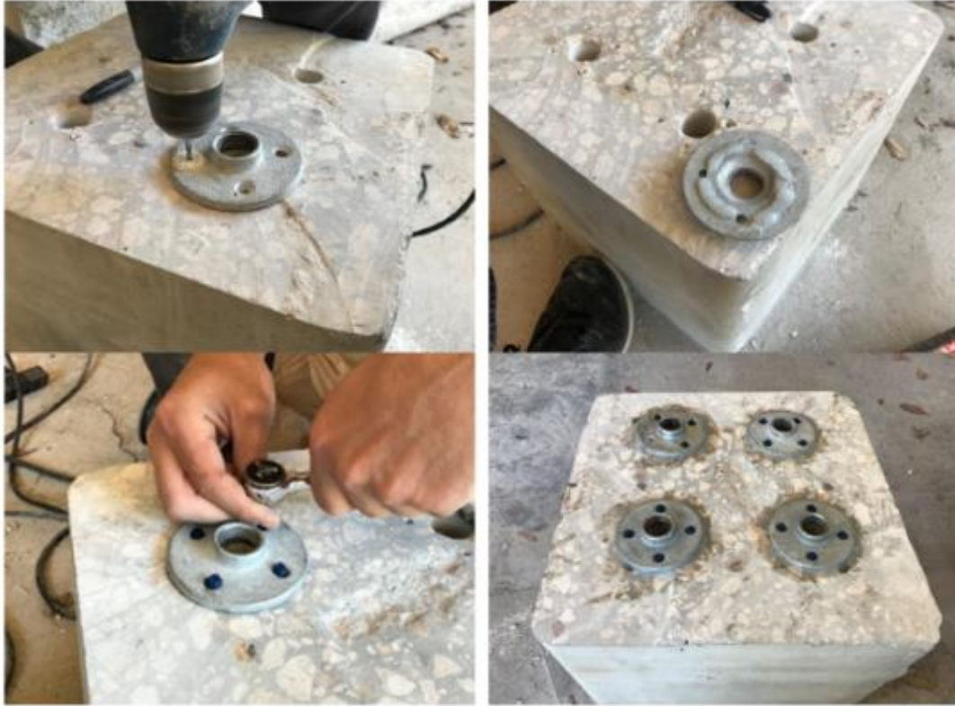
Figure 4-6: Predrilling holes into the concrete face (top left); Silicon applied to the bottom of the metal flanges (top right); Anchoring the metal flanges to the concrete face (bottom left); All flanges anchored and silicon placed around the flanges (right).
