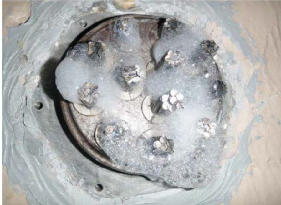
Figure 2-3: Impregnation fluid reported to successfully displace moisture from a tendon end opposite to the injection end. 47
