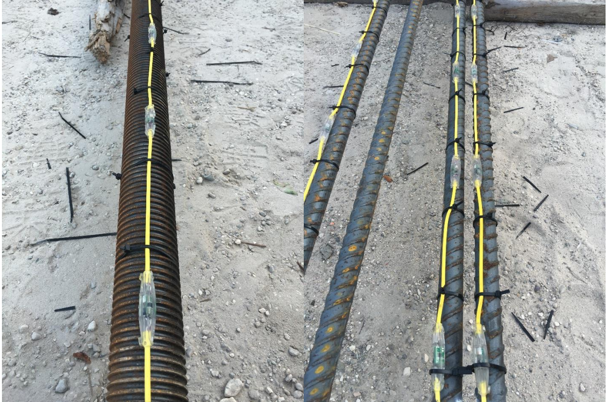
Figure 2.8 3-in center bars (left) and #11 center bars (right) instrumented with thermal wires.
