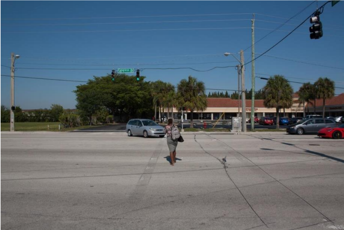
Photo 4-15 Crosswalk markings on S. Congress Ave. at the entrance to Palm Beach State College are faded
