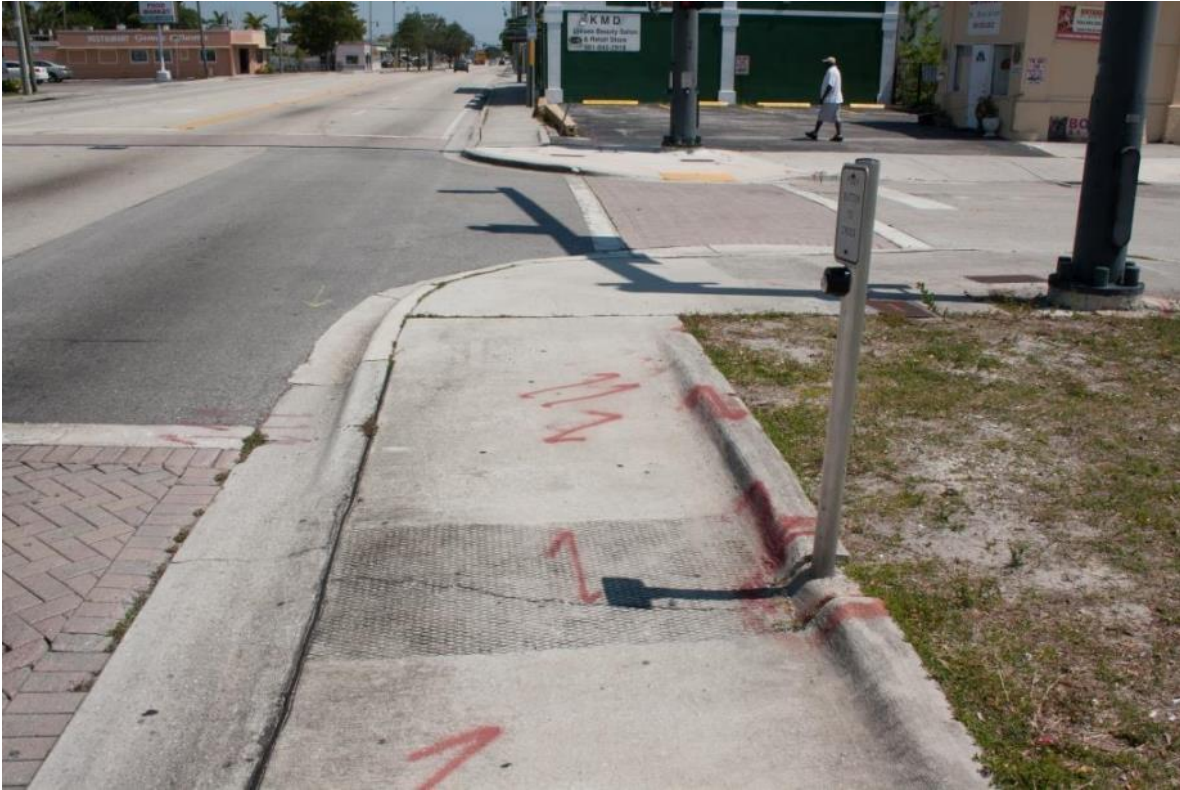
Photo 4-25 ADA tactile paver at Broadway and 40th Street is out of date
