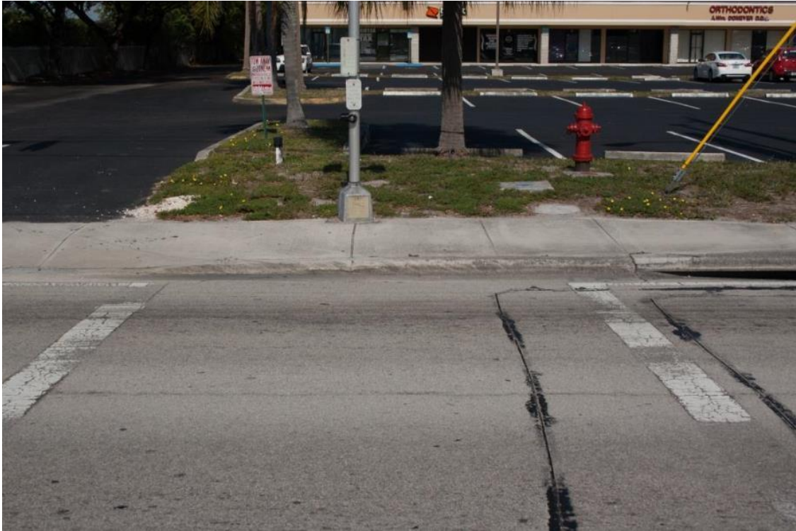
Photo 4-17 There is no ADA ramp on west side of S. Congress Ave. near the entrance to Palm Beach State College
