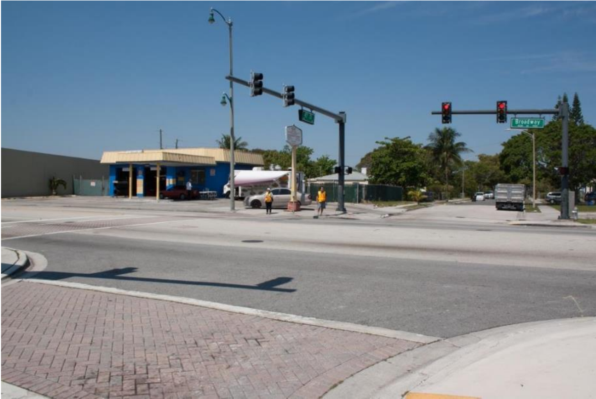
Photo 4-23 Brick pavers at Broadway and 40th Street have faded
